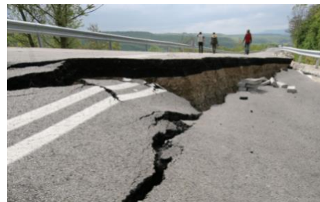
Earthquake damage to infrastructure can slow the return to normal operations. Image is courtesy of the USGS.
